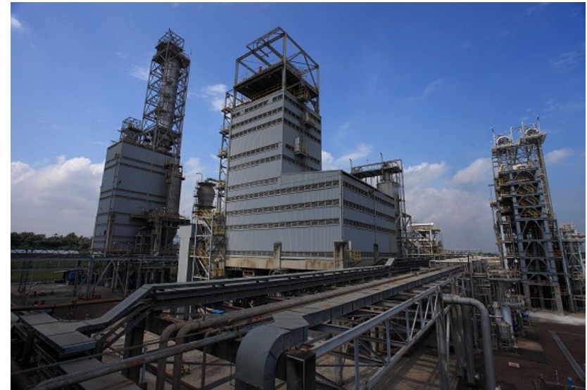
Existing PE plant in Cilegon with capacity 336 KTA with 1 train UNIPOL PE Technology 200 KTA and 1 train Showa Denko PE Technology 136 KTA
